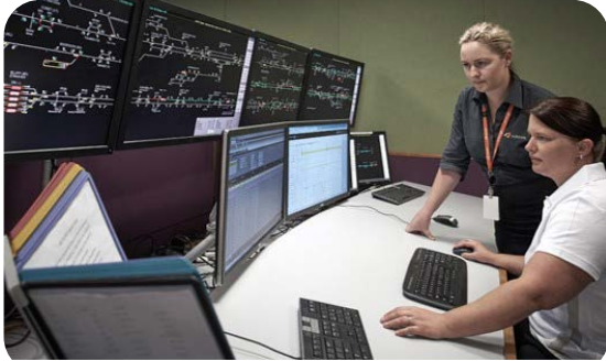
Rockhampton Control Centre
