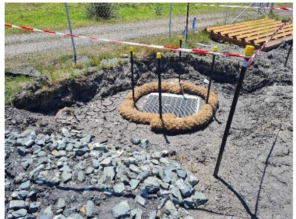
Figure 4: Stormwater inlet protection (March 2023)
