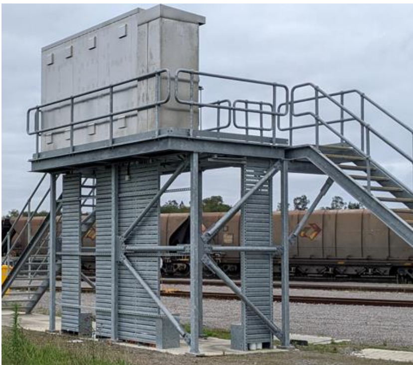
Figure 8.1 CMF main switchboard
