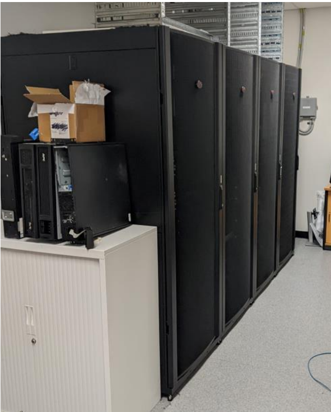
Figure 8.2 CMF communications room
