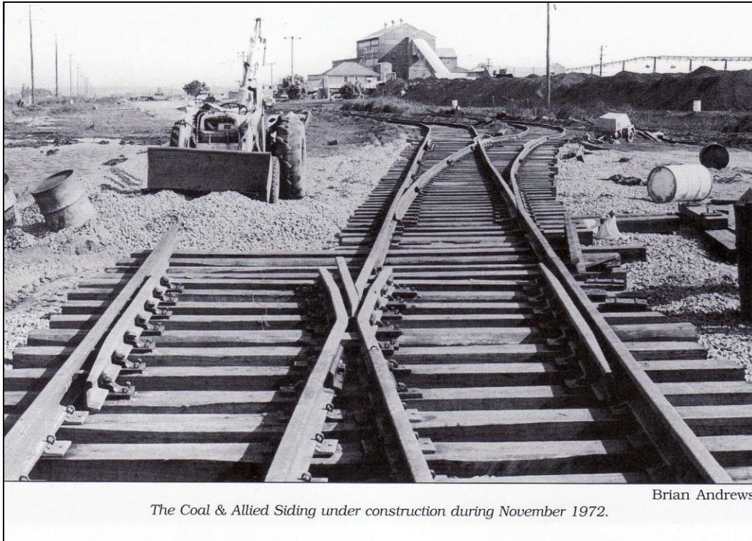
Figure 23. Coal and Allied siding under construction during November 1972. The Coal Preparation Plant and stockpiles can clearly be seen. Source: Brian Andrews, Coal, Railways and Mines
