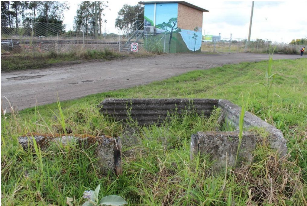
Figure 42. Ruin of former Hetton Bellbird weighbridge hut, showing doorway; the Great Northern Railway signal relay hut is elevated to guard against flood damage. Australian Museum Business Services
