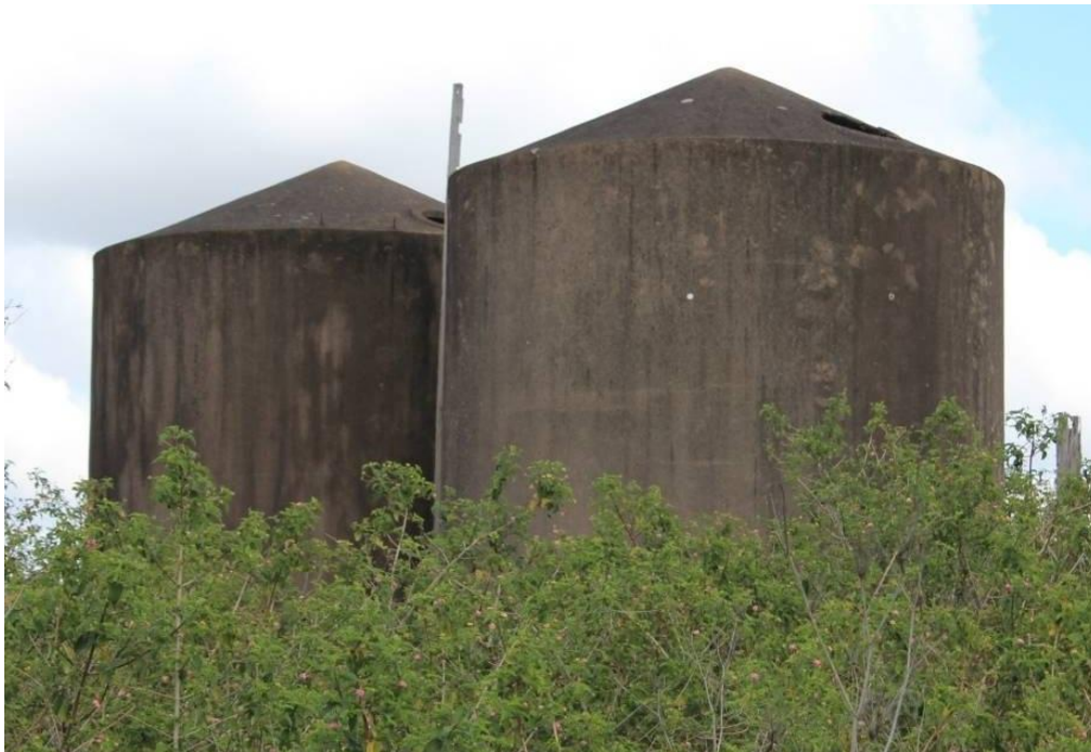
Figure 41. A closer view of the concrete feed silos. Australian Museum Business Services
